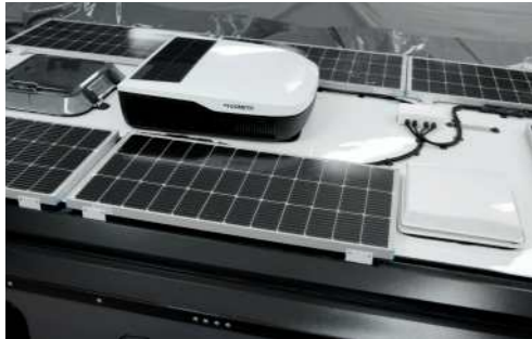
600W Roof Mounted Solar with 200AH Lithium Batteries
